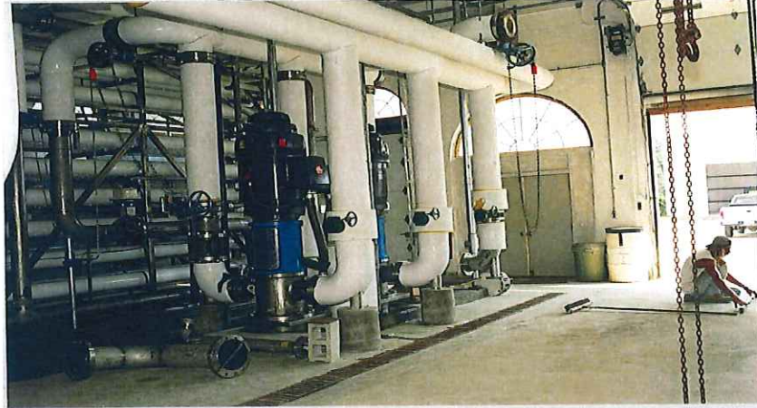
Desalination plant in Cape May City financed in part by the Drinking Water State Revolving Fund
