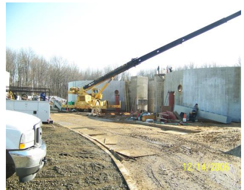
Mount Laurel MUA Elbo Lane Water Treatment Plant
