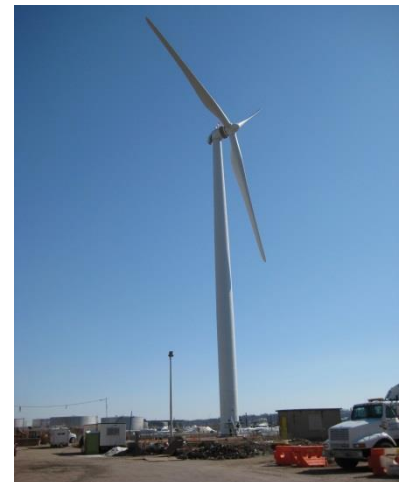
Bayonne MUA Wind Turbine for a Pump Station
