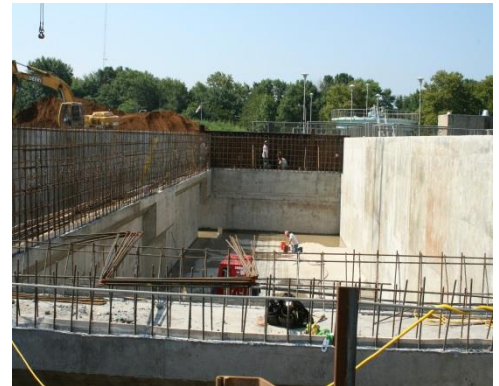
Township of Middletown Sanitary Authority Aeration Digester
