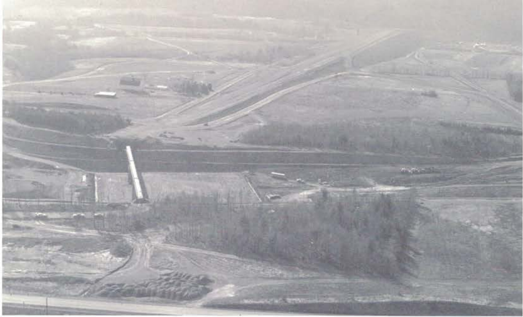
Corps of Engineers photograph shows final construction under way at Beltzville Reservoir in Lehigh Valley. Beyond spillway in foreground is the main dam structure.
