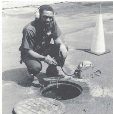
A Philadelphia Water Department repairman uses a Detect-A-Leak unit to listen to water main valves, fire hydrants and service lines to detect leak noise. Plugging the unit into a van-mounted computer allows the leak to be pinpointed with accuracy.
