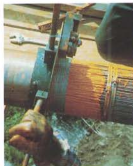
A worker rewraps the rehabilitated cables after the application of a rust-inhibitor paint. (Photo by Sandy Speers, NPS)
