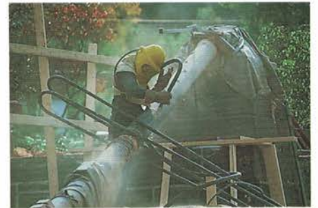
The structure is blasted with water and rounded glass beads to remove rust and dirt. (Photo by Sandy Speers, NPS)
