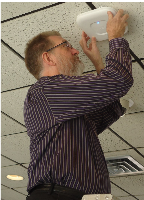
Senior Information Specialist Karl Heinicke inspects one of the DRBC building's wireless routers.
