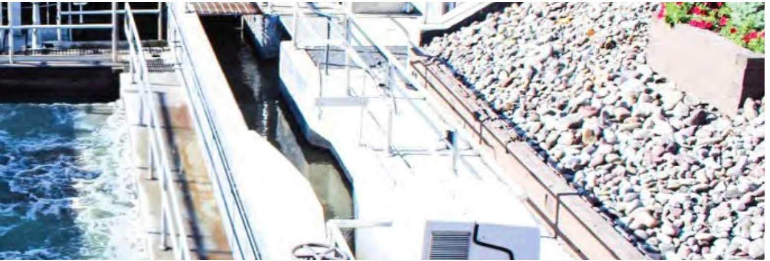
The flow metering and pre-aeration part of the Joint Municipal Authority of Wyomissing Valley's waste water treatment plant.
