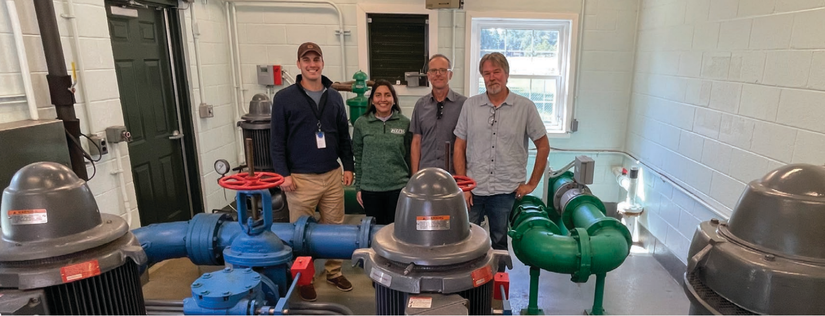
DRBC Project Review and Water Resource Planning staff toured the New Castle, Del., Municipal Services Commission.
