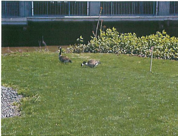
Photographs 4: Markers on the former landfill denoting areas that need repair
