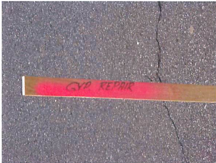
Photographs 5: Markers on the former landfill denoting areas that need repair
