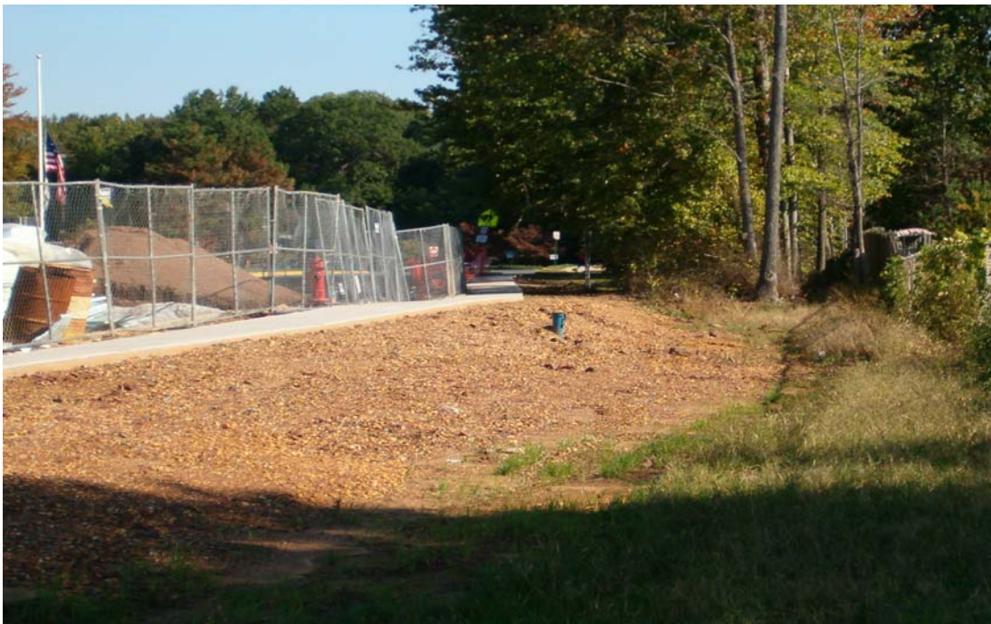
Photograph 4: Drainage swale to south of high school. Monitoring well in background. View facing northwest towards Raider Road.
