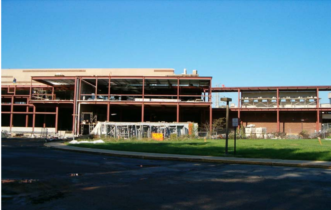
Photograph 1: View of new school addition from south side of North Brunswick Township High School (NBTHS).
