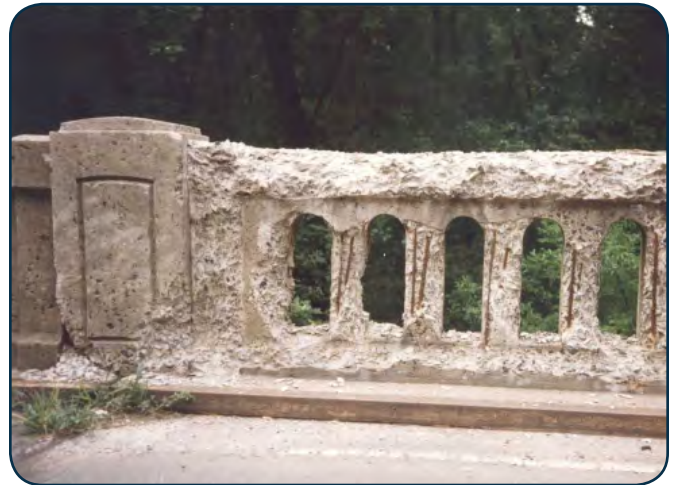
The reinforced concrete balustrade was severely deteriorated. (Courtesy of NJHPO).
