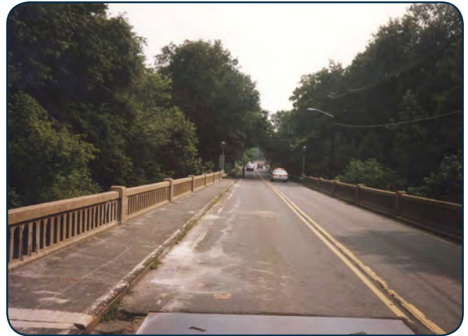
Millstone Causeway before superstructure replacement . Note the single sidewalk, perforated balustrade and historic light fixtures at the far end of the bridge. (Courtesy of NJHPO).
