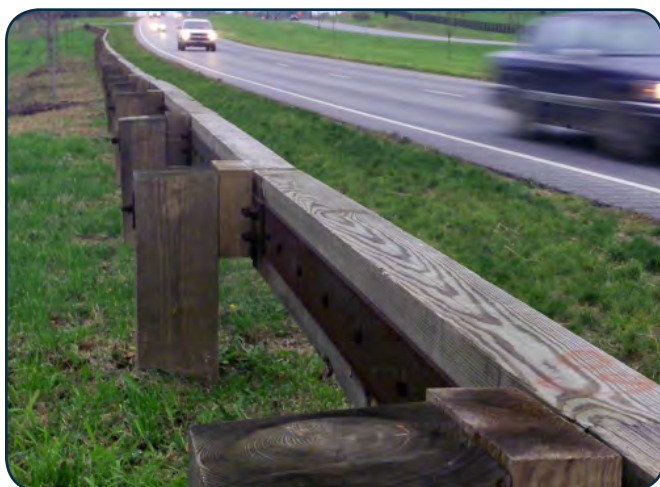
A reinforced guide rail along Paris Pike, a historic and scenic roadway in Kentucky. (Courtesy of Pars International.)
