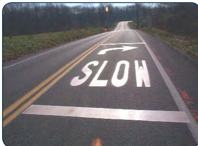
Use of thermoplastic pavement marking as an advance curve warning reduces the need for signs along the roadway. (Courtesy of the Federal Highway Administration.)
