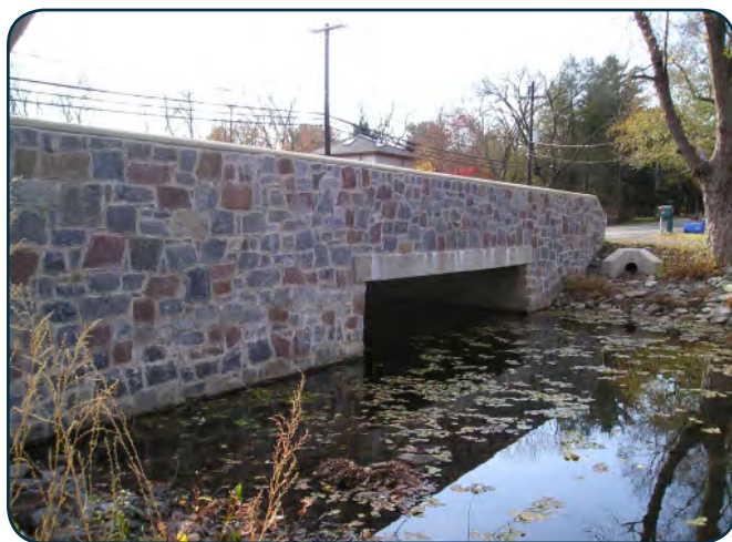
Stone from the historic bridge was used in this reconstruction, which was aligned on the original bridge footprint. (Courtesy of NJDOT.)
