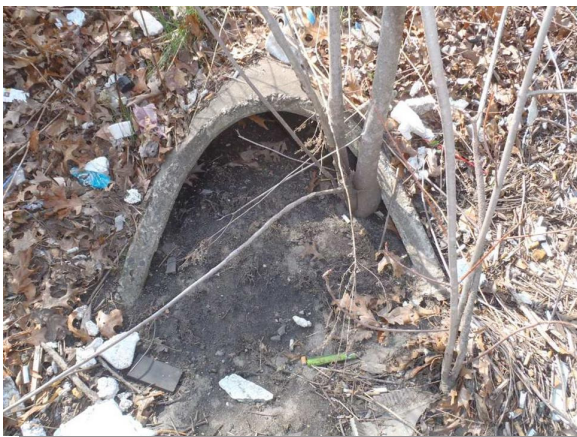
Clogged inlet pipe in urgent need of maintenance
