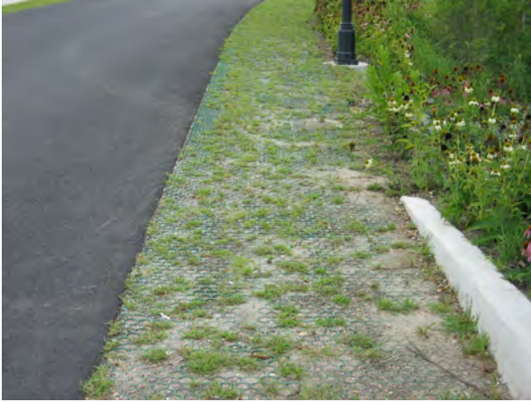
Race Street in Vincentown Historic District. The interlocking geogrids will allow grass to grow yet have the strength to act as a sidewalk and shoulder while allowing water to percolate
