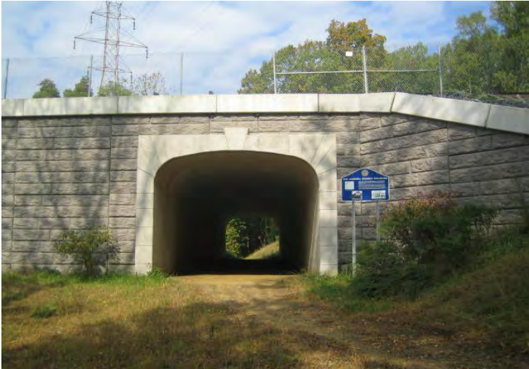
Rt. 130 over the historic Kin-kora Branch Railroad includes a culvert for animal and human access
