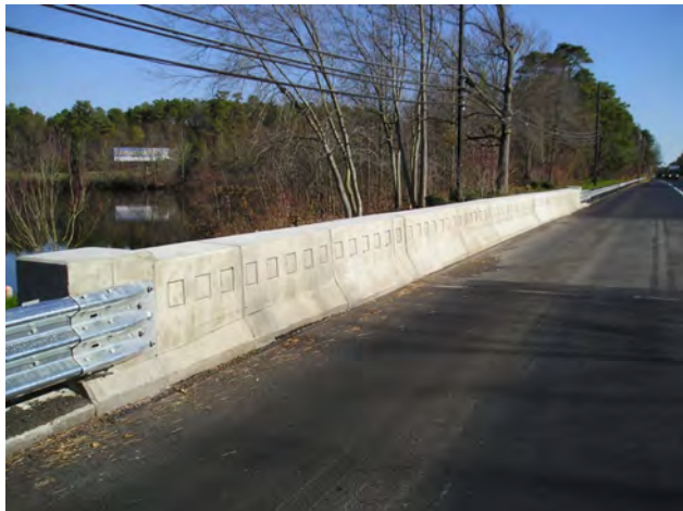
Rt. 70 Rockefeller Memorial High- way Historic District (inboard and outboard treatment of a Jersey Barrier)
