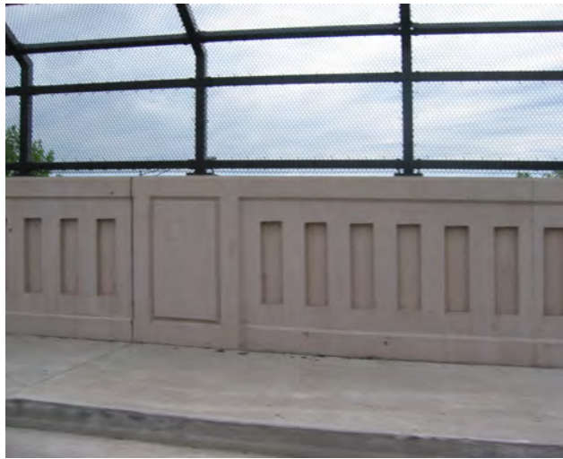
Southard Street bridge over Rt. 1 and the Camden and Amboy Railroad Historic District and Delaware and Raritan Canal Historic District
