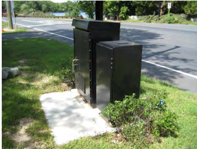
Rt. 47 screening of the powder coated signal appurtenances within Dennisville Historic District
