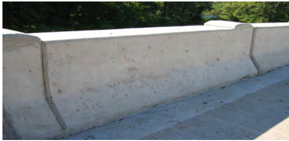
Rt. 31 Readington Township Rowland's Mills Historic District (outboard and inboard treatment of Jersey Barrier; note the pylons)
