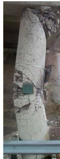
(b) Minnesota I90 bridge accident (2003).
