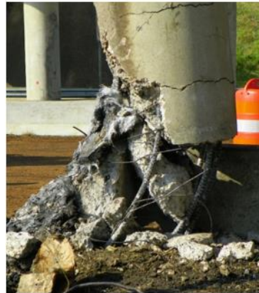
(b) Texas I45 bridge accident 2014.
