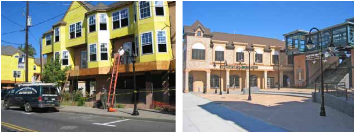
Transit-supportive housing under construction in South Amboy (left) and mixed use development at the station (right).
