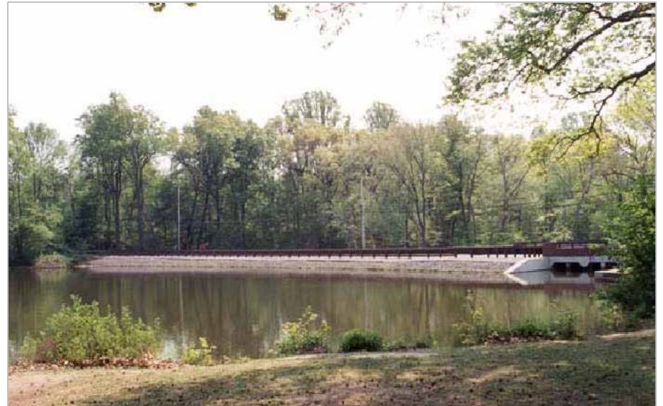
Brown steel guiderail on Pond Road in Freehold Township blends into the landscape. Image source: Monmouth County, Design Guidelines for Monmouth County's Scenic Roads
