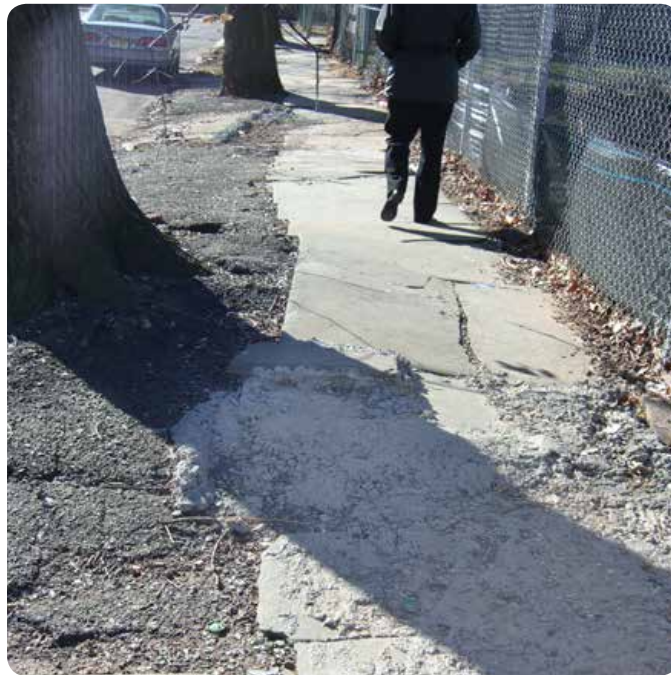
Poor example: This poorly maintained sidewalk is a hazardous impediment for pedestrians and is likely impassable for a wheelchair. It sends the message that this space is not cared for. Image: The RBA Group
