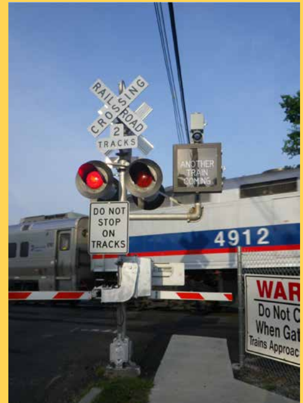
“Another Train Coming” system installed at Plauderville Station. Image: Marco DeSilva, Volpe Center
