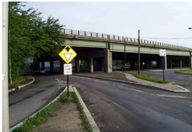
The crosswalks are unmarked and curb ramps absent at this ramp, located one block from an elementary school in Camden. Image: Cambridge Systematics
