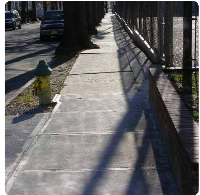
Good example: This well maintained sidewalk, which shows a recent repair, is safe for passage on foot or in a wheelchair. It sends the message that this space is highly cared for. Image: The RBA Group
