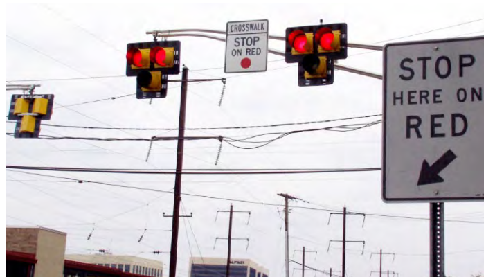
NJDOT installed a pedestrian hybrid beacon, or HAWK signal, at Route 27 in Woodbridge near the Metropark Rail Station. Image: NJDOT
