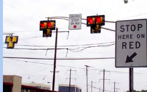
Pedestrian hybrid beacon on Route 27 in Woodbridge near Metropark Station. Image: NJDOT
