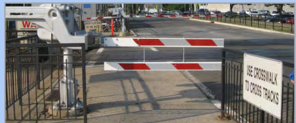
Pedestrian gate with “gate skirt” being tested at the Aberdeen-Matawan Train Station. Image: The RBA Group
