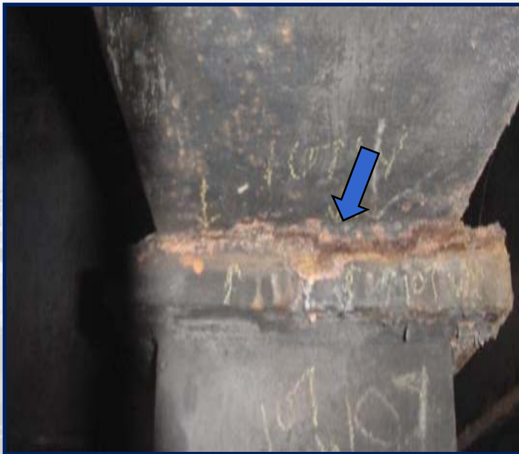
Cracked Weld at Column / Pier Cap Connection
