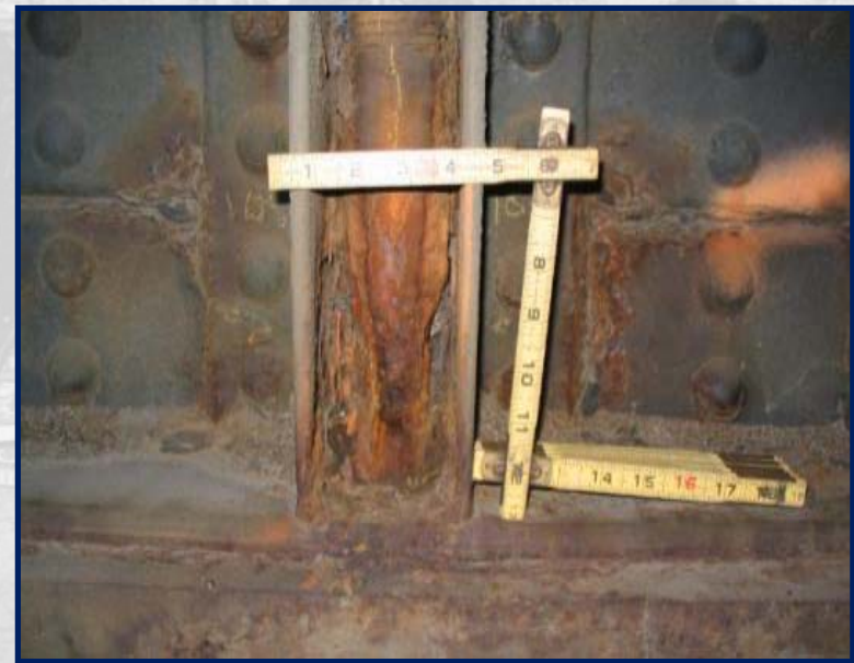
Up to 50% Anchor Bolt Section Loss at Base of Column for Pier Bent
