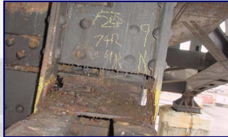
Up to 50% Section Loss Hanger Vertical Members
