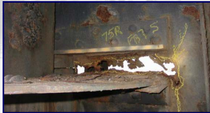
Up to 100% Section Loss Floorbeam Member
