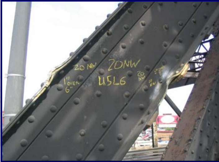
Vehicular Impact to Diagonal Member
