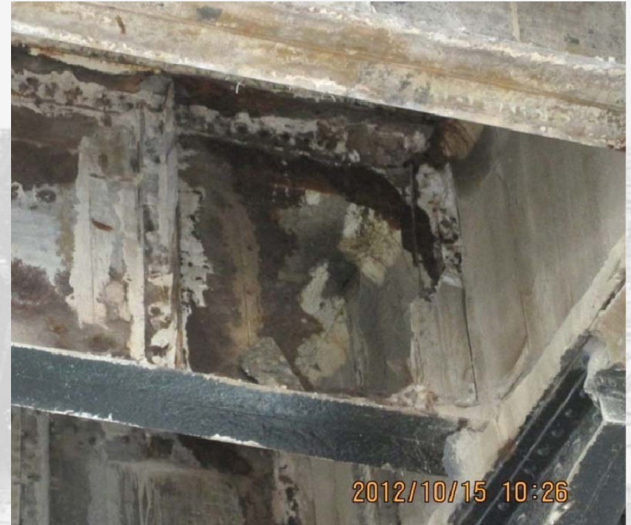
Hole in stringer with entire end panel missing
