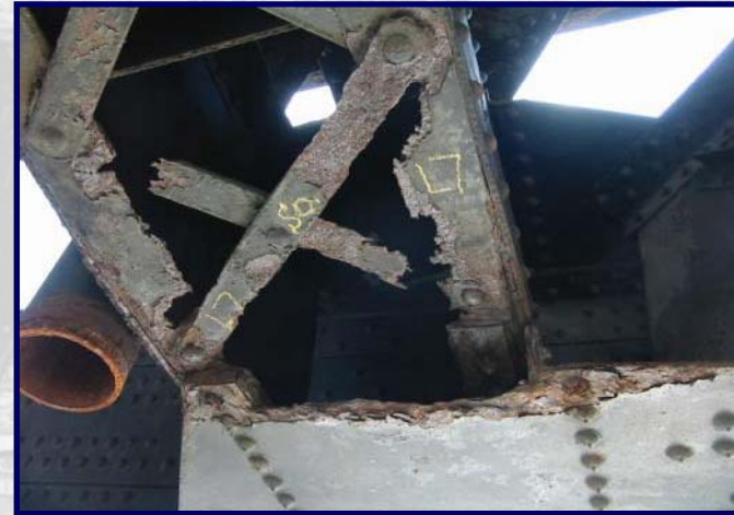
100% Loss to South Truss Lacing Bars and Horizontal Legs of Bottom Angles
