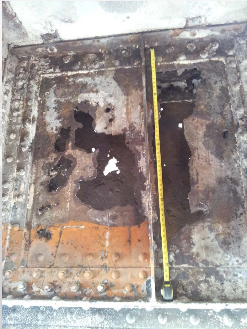
Holes in adjacent web panels
