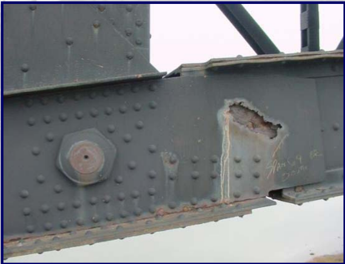
Holed-Through Gusset Plate in Lower Chord
