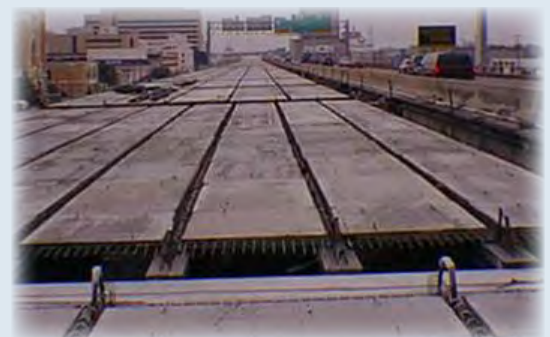
Precast concrete panels similar to what will be installed on the skyway
