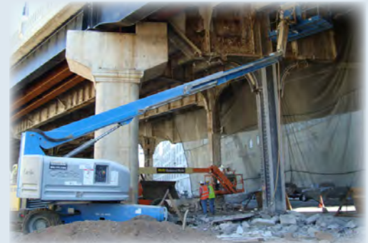
Showing removed concrete on front right column; concrete still encases column in middle
