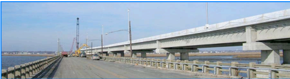
Demolition work on existing Rainbow Channel Bridge with newly constructed Rt. 52 Causeway in the background (Contract A)
