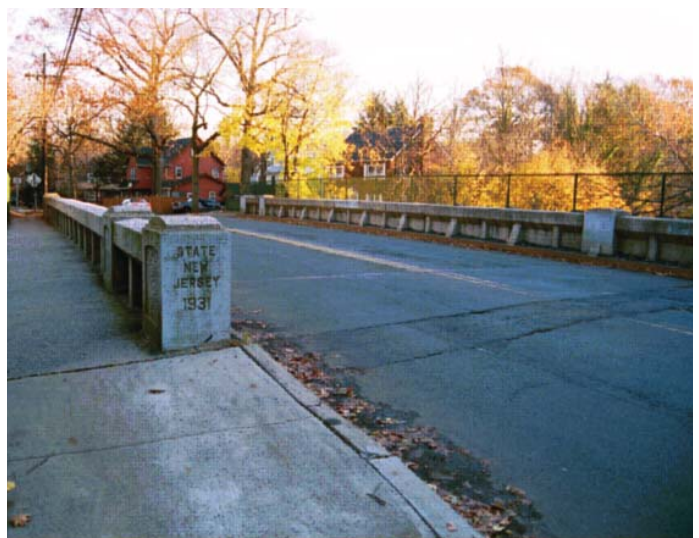
This bridge in Teaneck was constructed in 1931 and continues to serve local residents.
