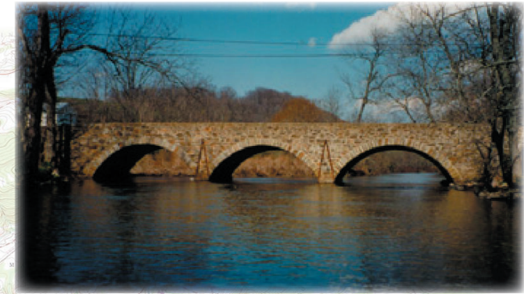
This existing stone arch bridge over the Musconetcong River could serve as a model for future context sensitive design in the corridor.
