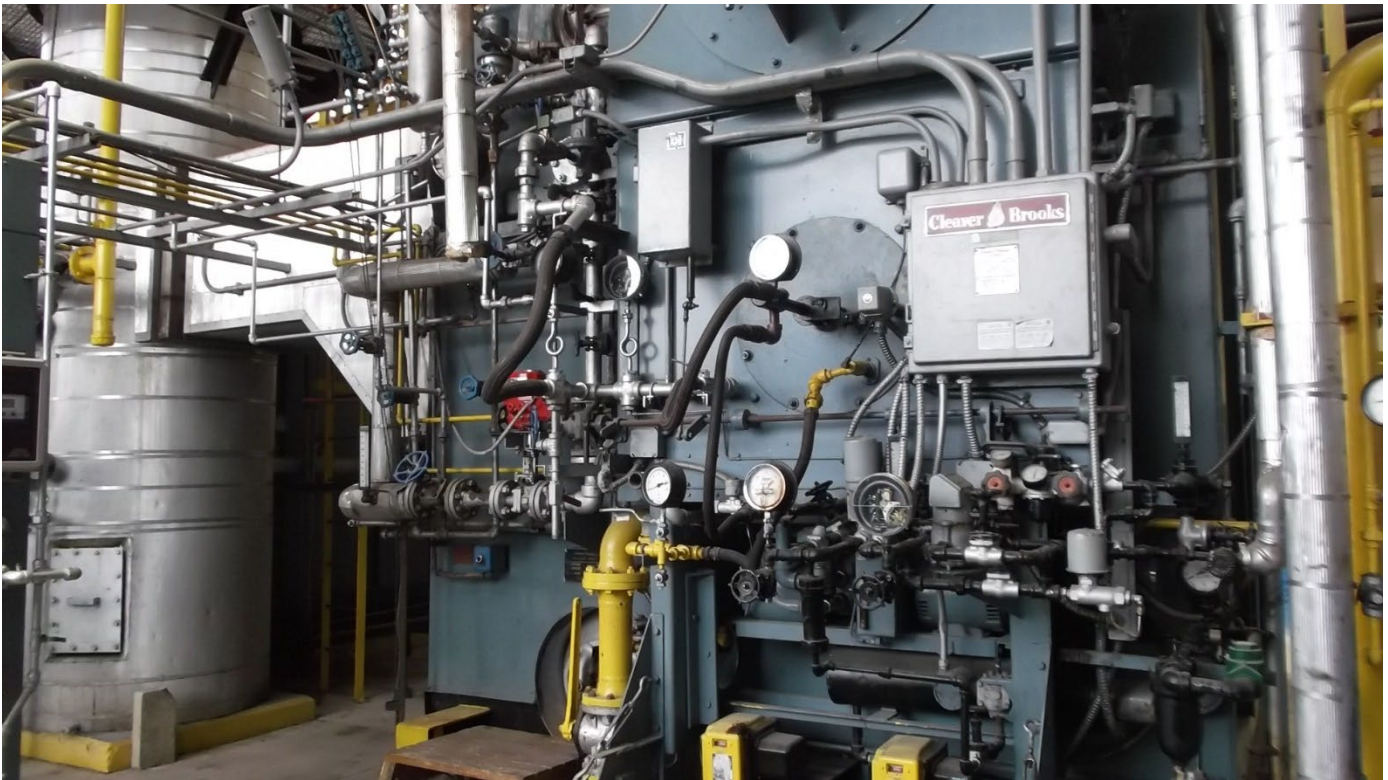
Boiler House EXHIBIT 'C'
