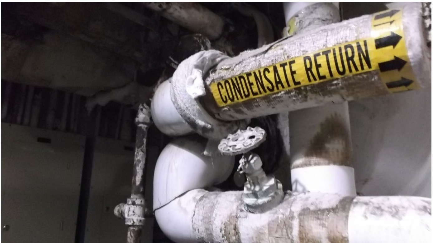
Typical shell and tube heat exchanger for domestic hot water.
