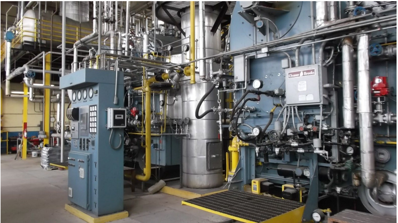
Boiler House EXHIBIT 'C'
